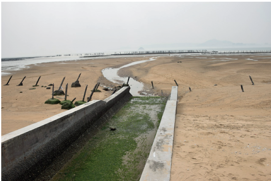
Figure 4: The 'jetty effect' at the Zhongdun Outlet project (Source: © Wen-Hua Huang, 3 April 2016)
